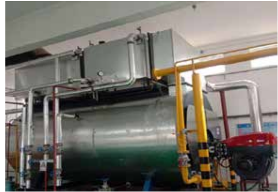
Boiler Heat Recovery 鍋爐餘熱回收設備
